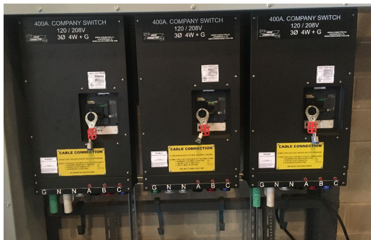
Photo of lighting company switches
