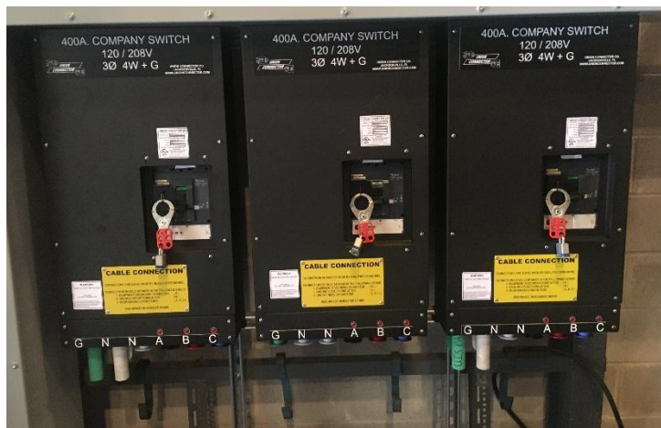
Photo of lighting company switches
